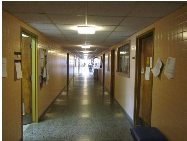
A Jewett Hall corridor, an inflexible building layout and construction type that is difficult to repurpose.
