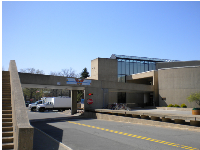
The elevated spine connecting to the Williams Center above Old Main Drive. The spine remains a prominent physical element of the campus and a symbol of the Pei-Cobb Master Plan, but is in a severely deteriorating condition.
